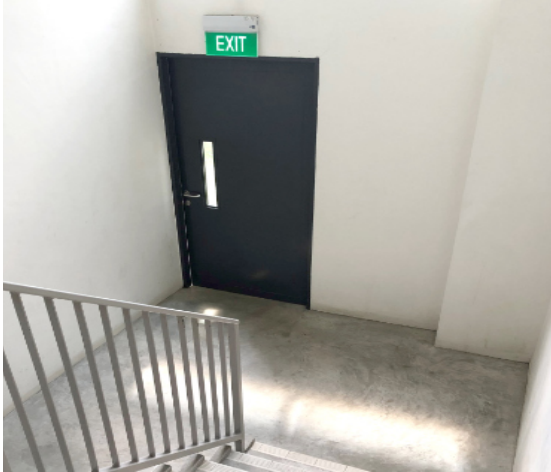
Exit sign placed over the exit door
