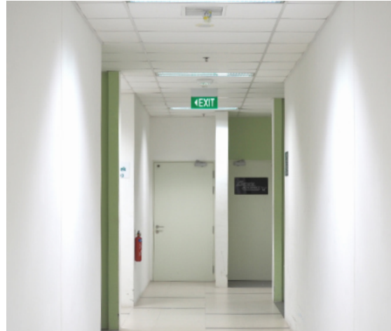
Directional exit signs in long corridors
